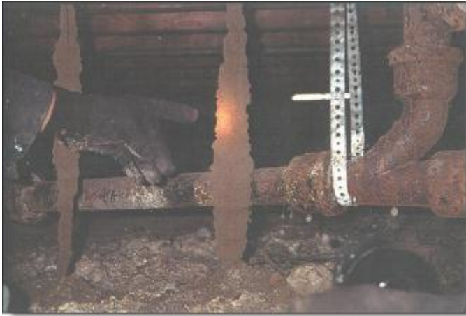
Shelter tube in center of living room # 1
